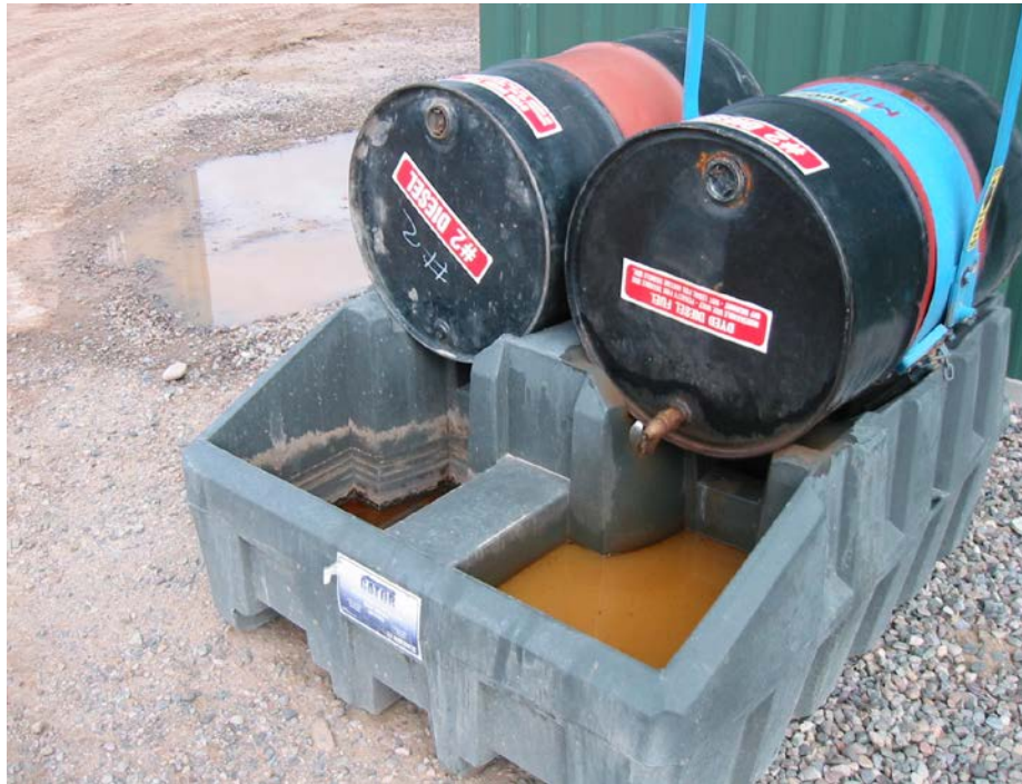
Drum Caddy Secondary Containment
