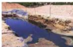
Torn pit liner. Photo courtesy of Earthwork
