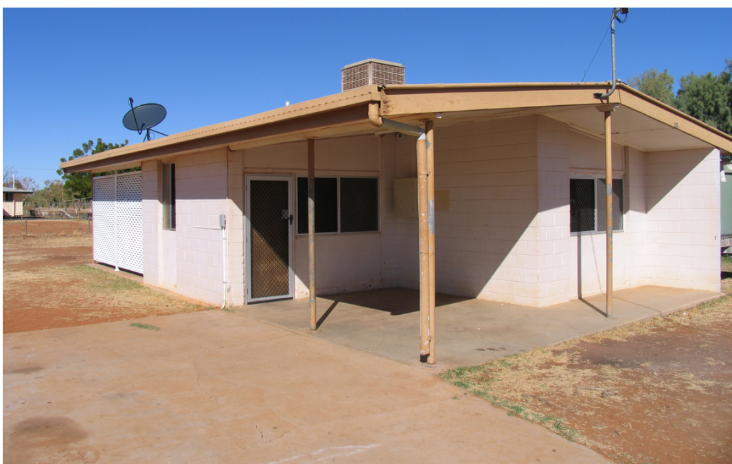
Figure 36: Managed by the Queensland Government, this house in Dajarra was vacant in June 2008. It had been inundated by creek flooding the previous year, with the tenants moving to the Jimberella Hall. (Photo by Tim O'Rourke)
