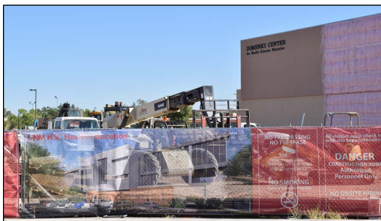
This photo taken on Sept. 15, 2016, shows the continued construction in the area west of the Domenici Center. This expansion of the Domenici Center was made possible by GO Bond B, which New Mexico voters approved in 2014.
