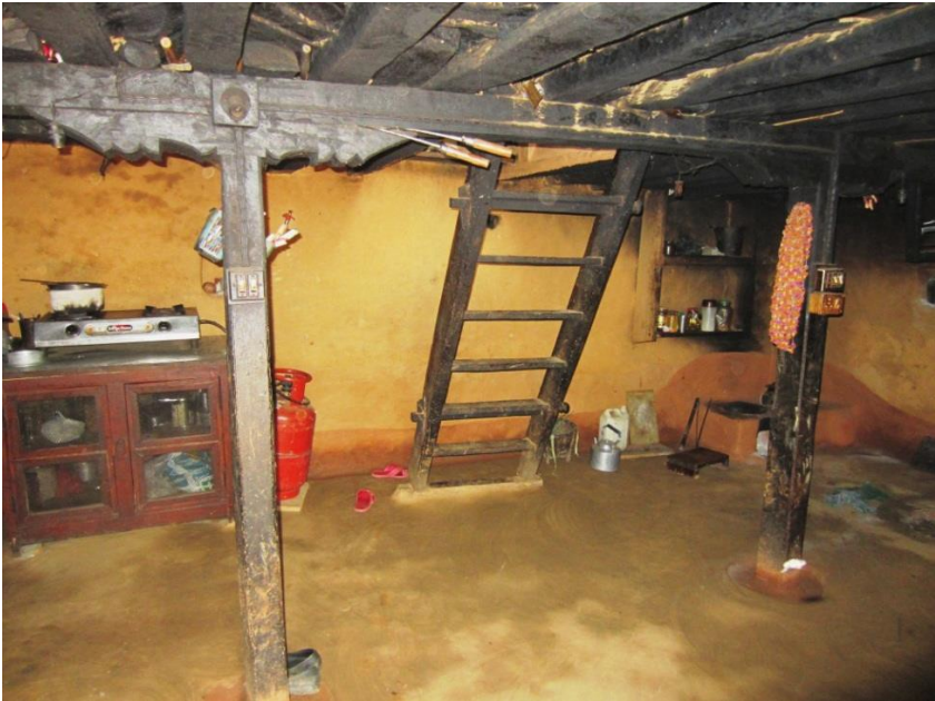
Figure 4: Smoke blackened ceiling
