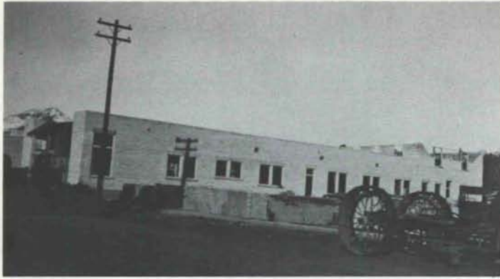
fig. 5 east wing with roof and beginning the second story in the center. Note heavy construction vehicle on the right.
