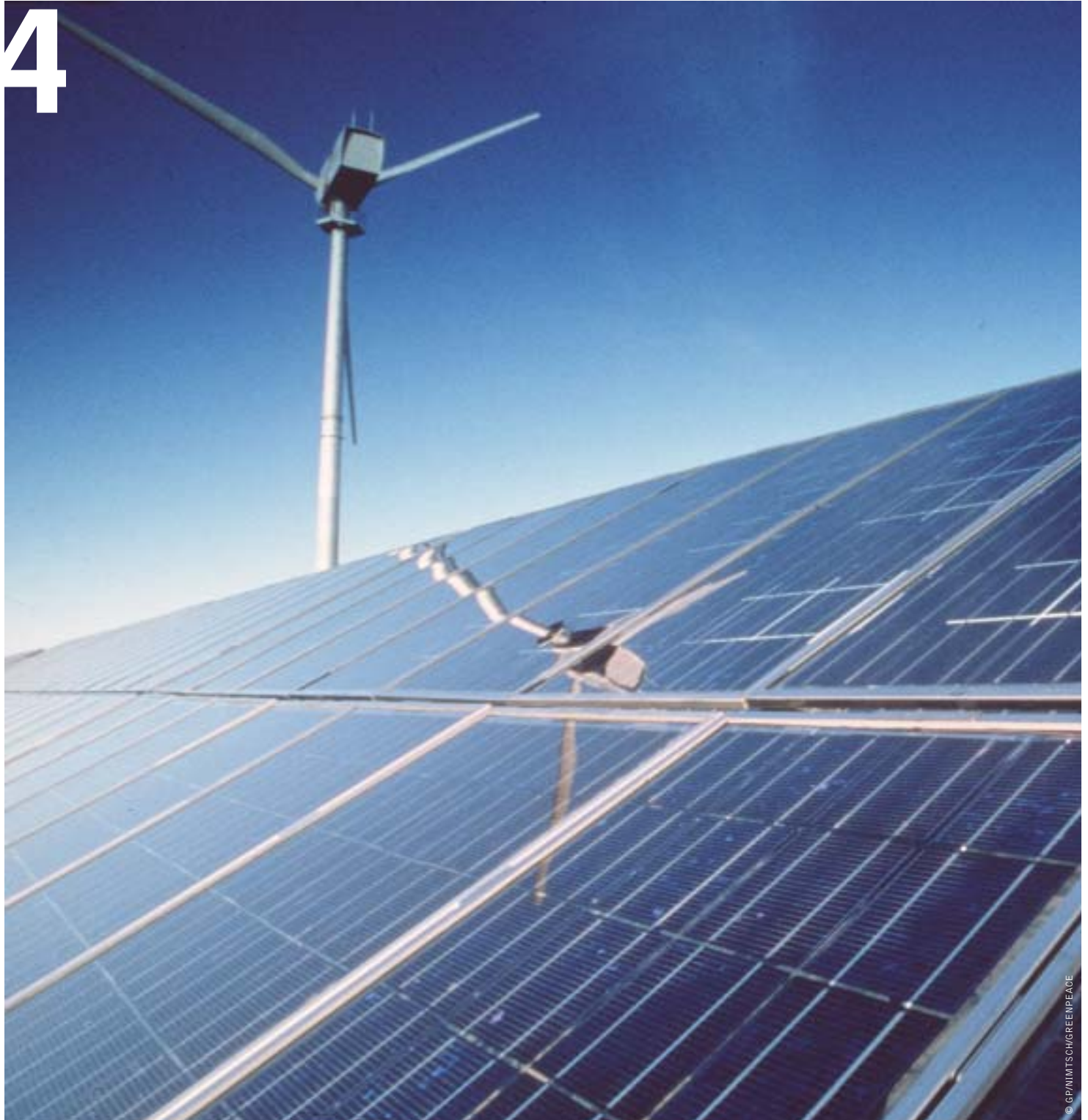
image SOLAR AND WIND-FACILITY NEAR ROSTOCK, GERMANY.
