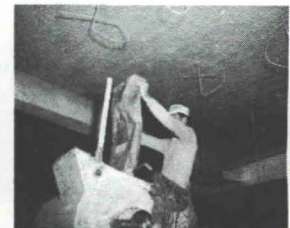
2 Finished fireproofing treatment presents pleasing surface and texture. Photos taken at Bell Telephone Co. Building, Pittsburgh, Pa.
