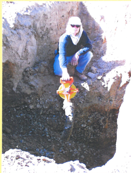
System drainline terminating at the seepage pit.
