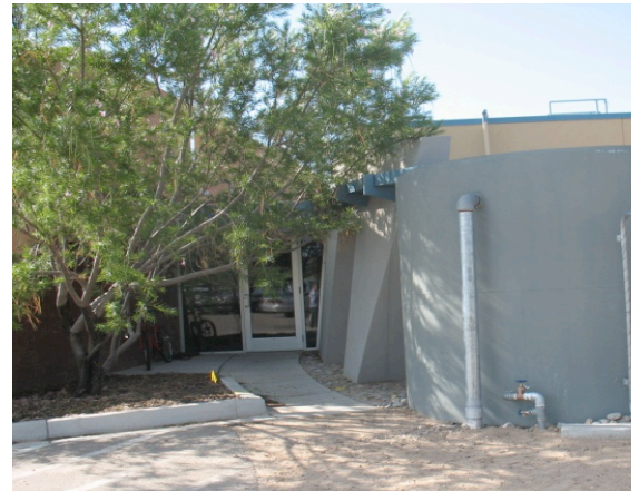
Figure 13: Cistern at SCAFCA offices, Rio Rancho, NM.
