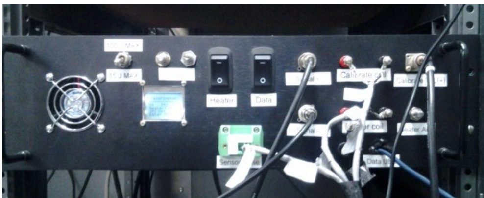
Figure 4.2.10. Calorimeter control panel.
