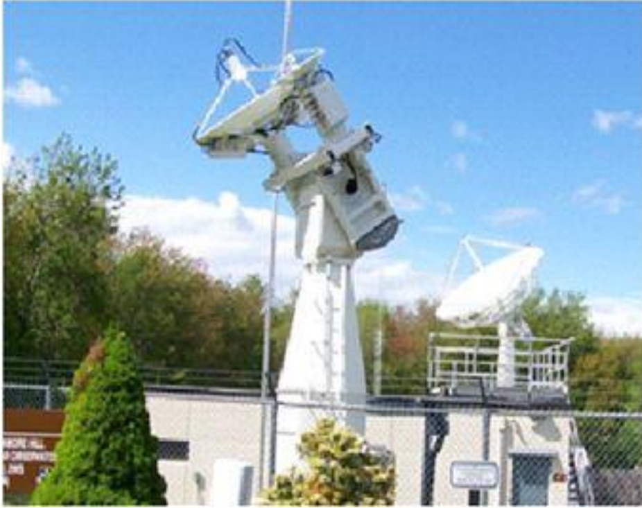
Figure 5: RSTN installation antennas.
