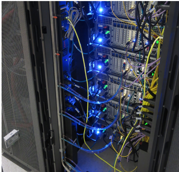
Figure 4: Image of the manifolds mounted in rack. Orange and black rubber caps block off the stub outs not in use.
