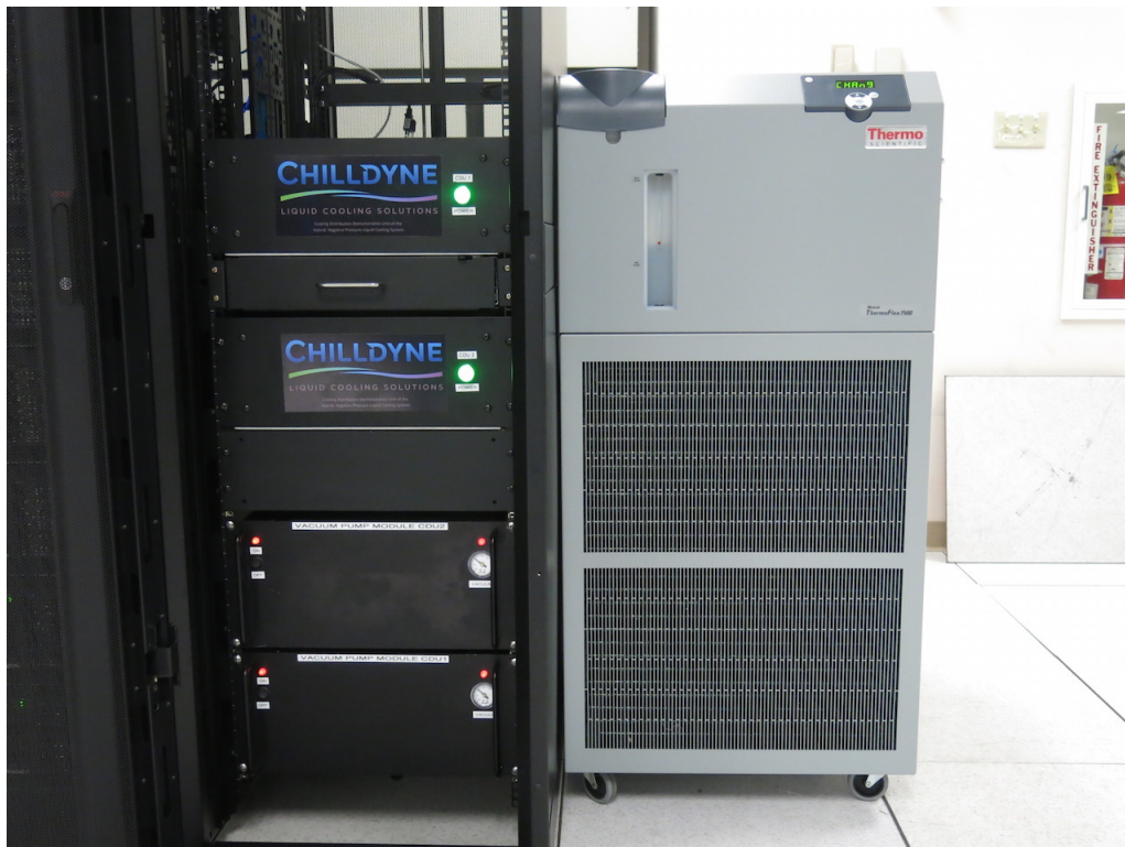
Figure 3: Image of the CDUs with vacuum pumps (left), and standalone chiller (right).
