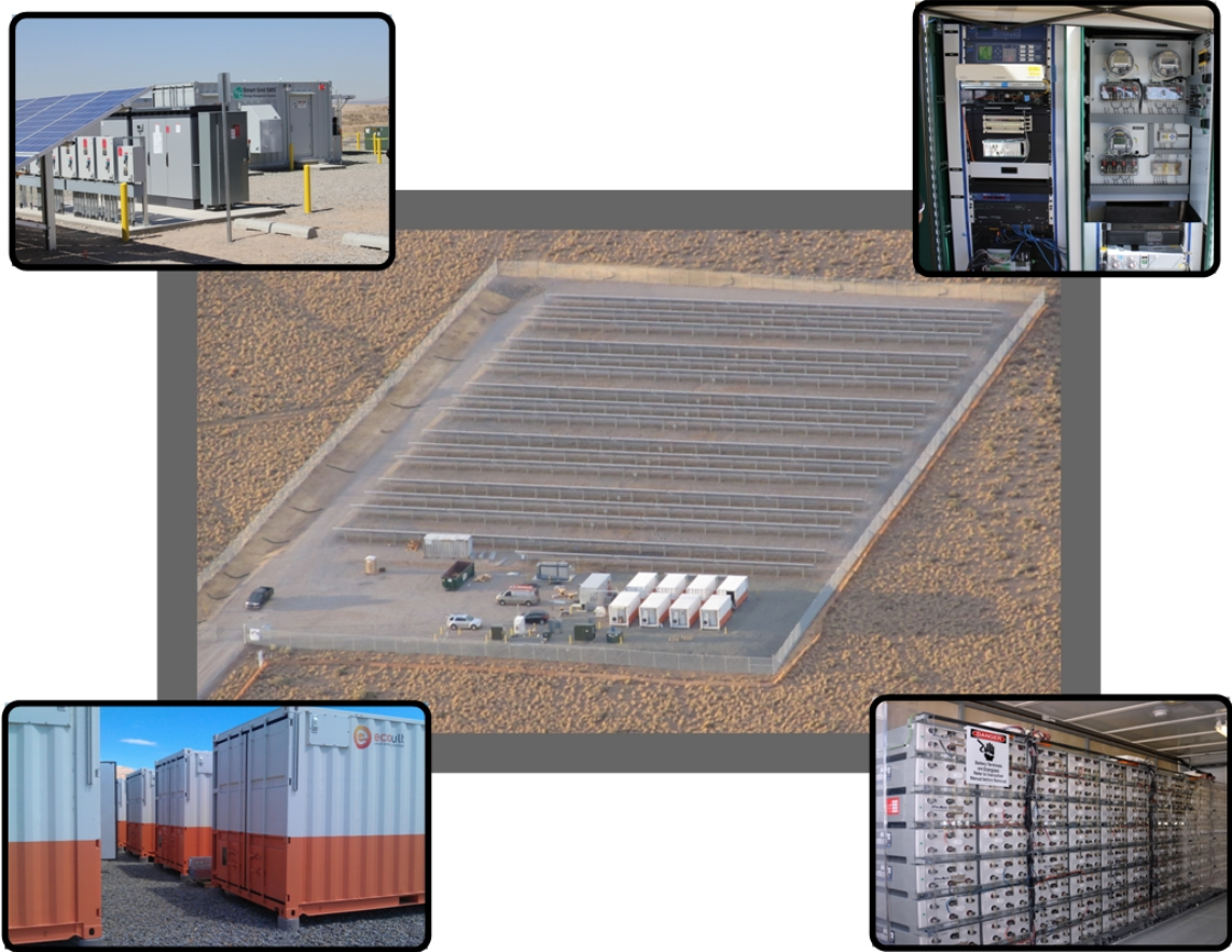
Figure 1.1: Prosperity Energy Storage Project site and battery energy storage equipment.
