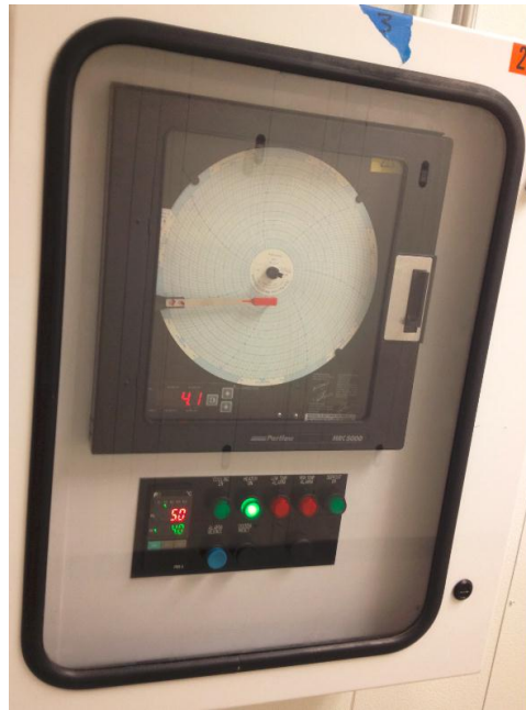
Figure 3.4.6.1 Control system of the freezer room
