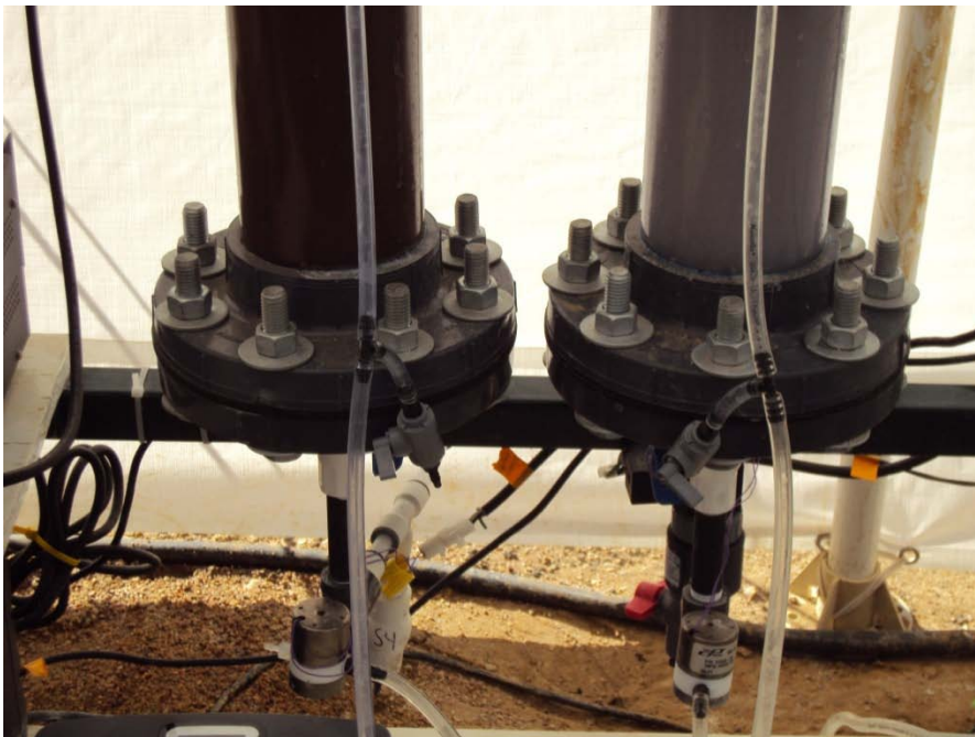
Figure 53: Solenoid Valves at Bottom of Columns
