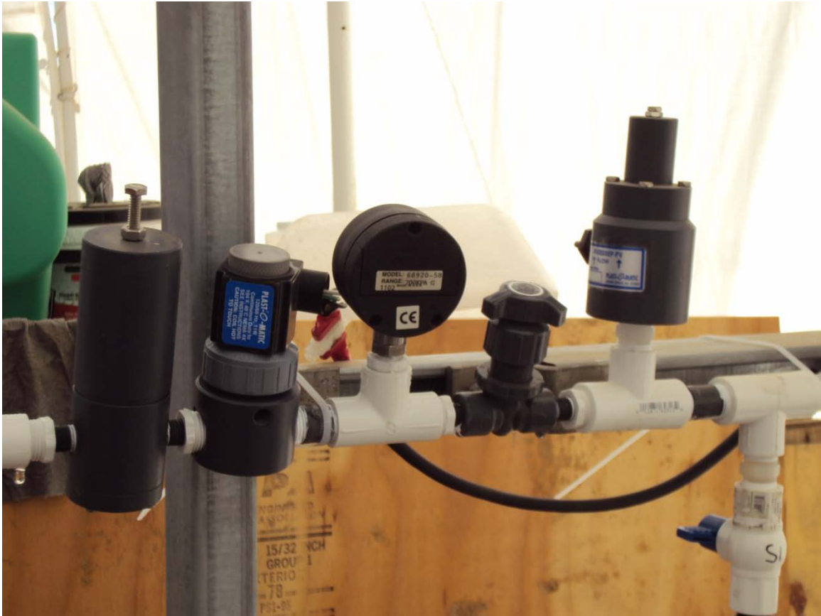
Figure 54: Control Sequence at Pilot Input including Pressure Reducer, Solenoid Valve, Pressure Gauge, Needle Valve, and Pressure Relief Valve
