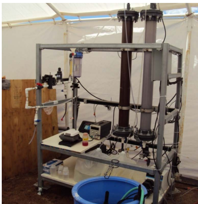
Figure 50: Pilot Equipment on Site
