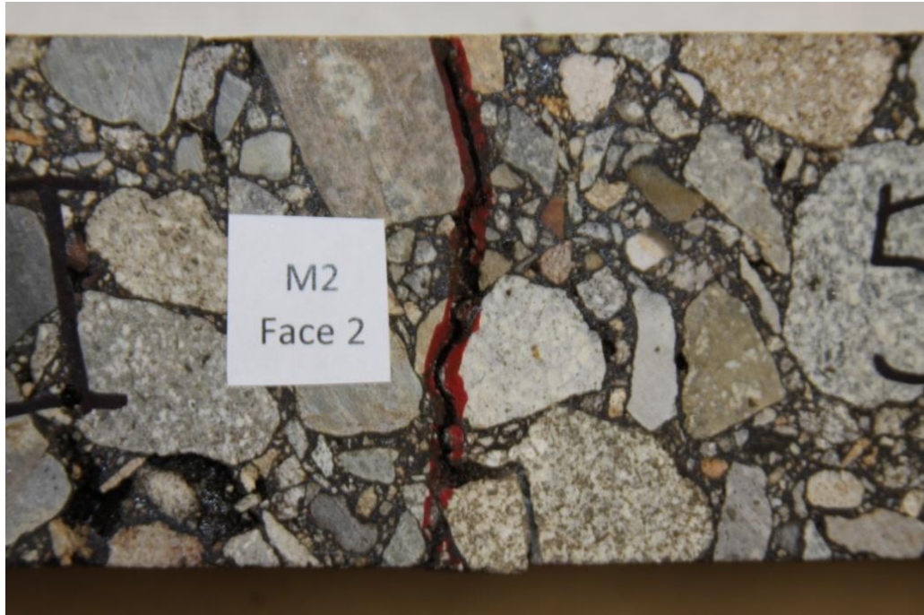
Figure 6.3 Fatigue Cracking in HMA Beam Sample SP-II-M2
