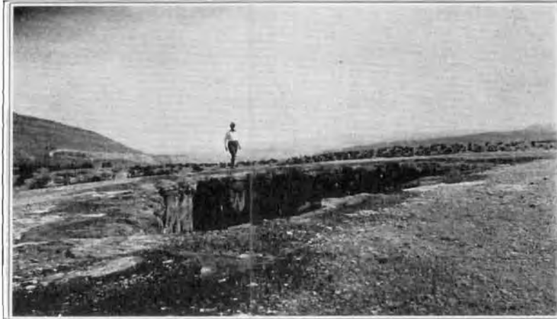
Figure 11. Another "crater." Water, which recently flowed over the top, now stands some 25 feet below the rim.
