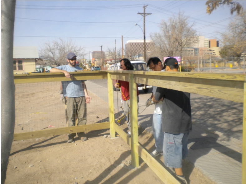
Barelas neighbors constructing a community garden next door to the neighborhood senior center and community center.
