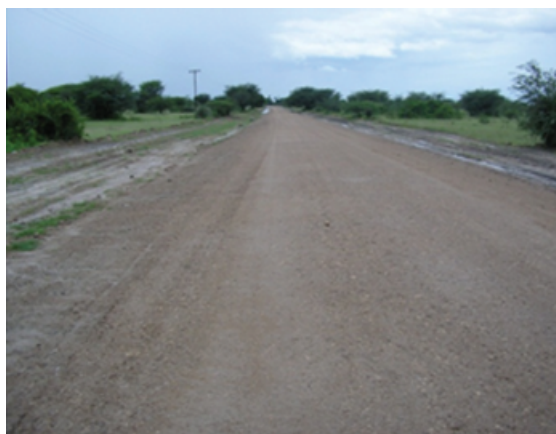
A major gravel road saturated with moisture
