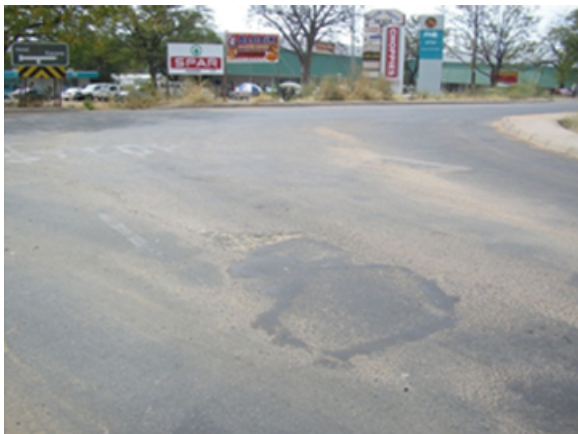
Paved road with defects
