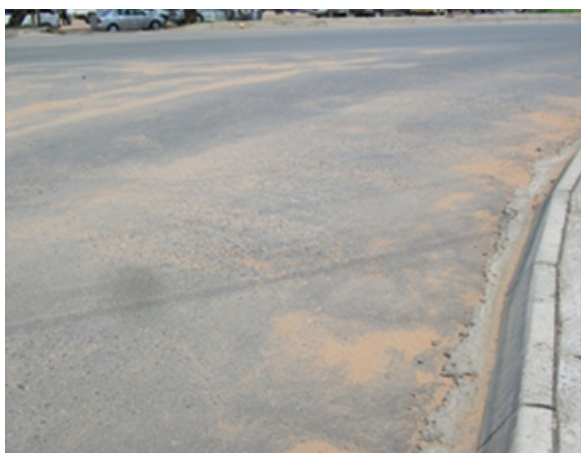
Paved road with defects
