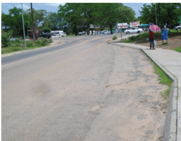
Bus bay with defects
