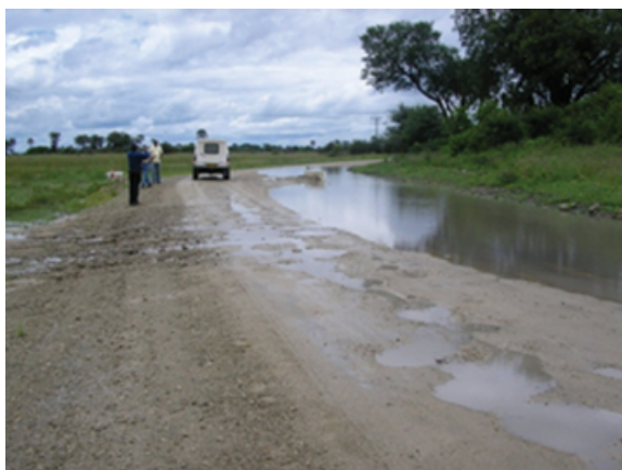
Gravel road and effect of bad drainage
