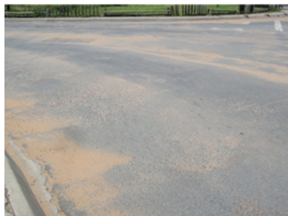
Paved road with defects
