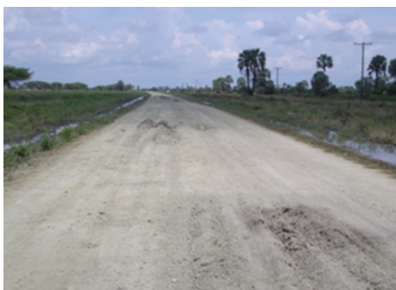
Gravel road with defects
