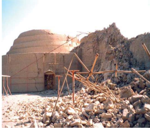
Figure A.5: Southern elevation of the Ice House (Ice maker), after the earthquake. The dome was reconstructed between 1974 and 2003; the original earthen walls survived the seismic forces (9EMS) with a vertical crack near the entrance in spite of the additional loading from the dome (Source: H. Darejati)
