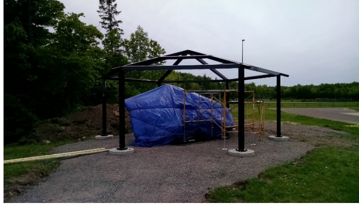
Figure 5: Lake Copper covered by blue tarp placed on engineered stand with construction of pavilion underway.
