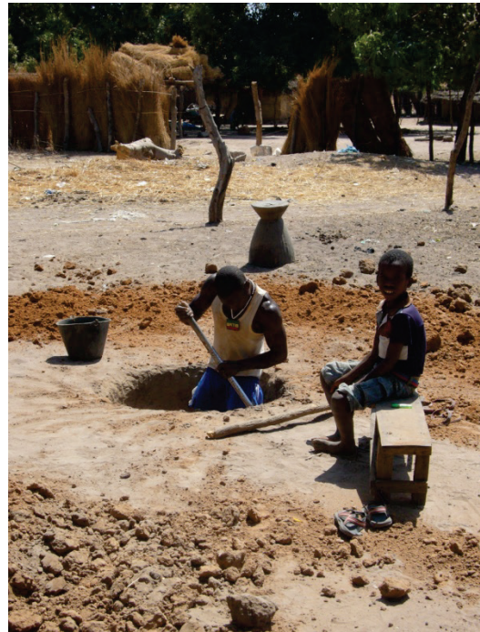
Figure 3. A man in Teyel, Kolda, Senegal digs a new well. Photo credit: Barbara Michel
