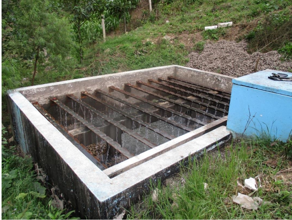
Figure 1.6: Trickling filter in Palmira WWTP. Photo by author.
