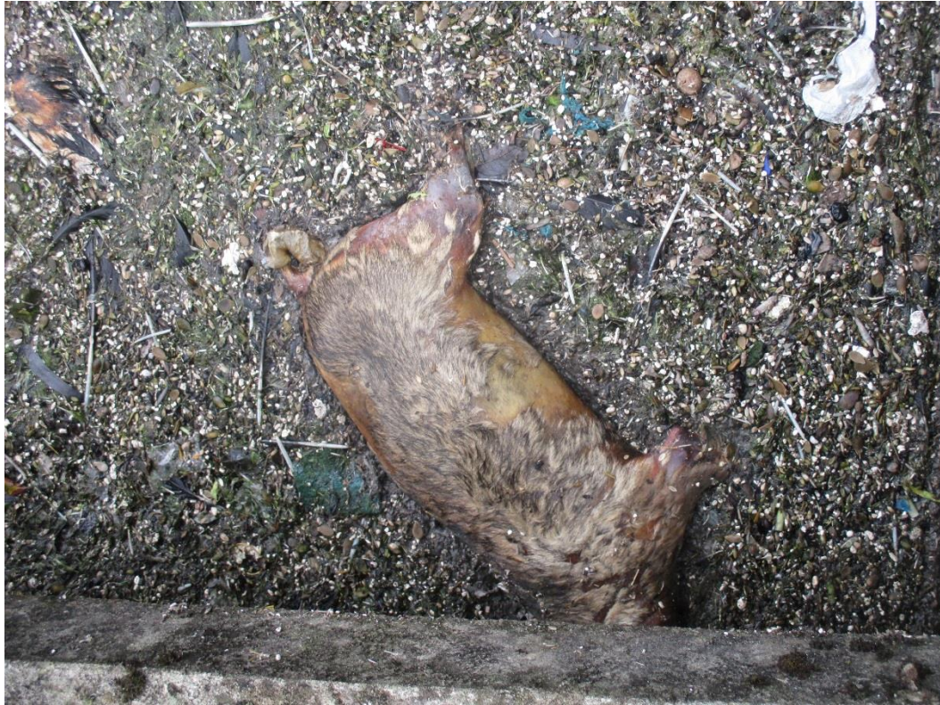
Figure 3.1: Dense scum layer in Imhoff tank with dead animals
