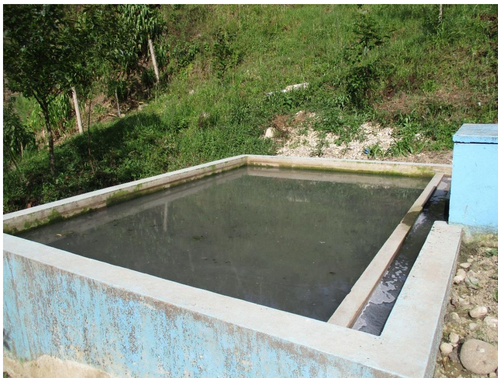
Figure 3.2: Clogged trickling filter in Palmira
