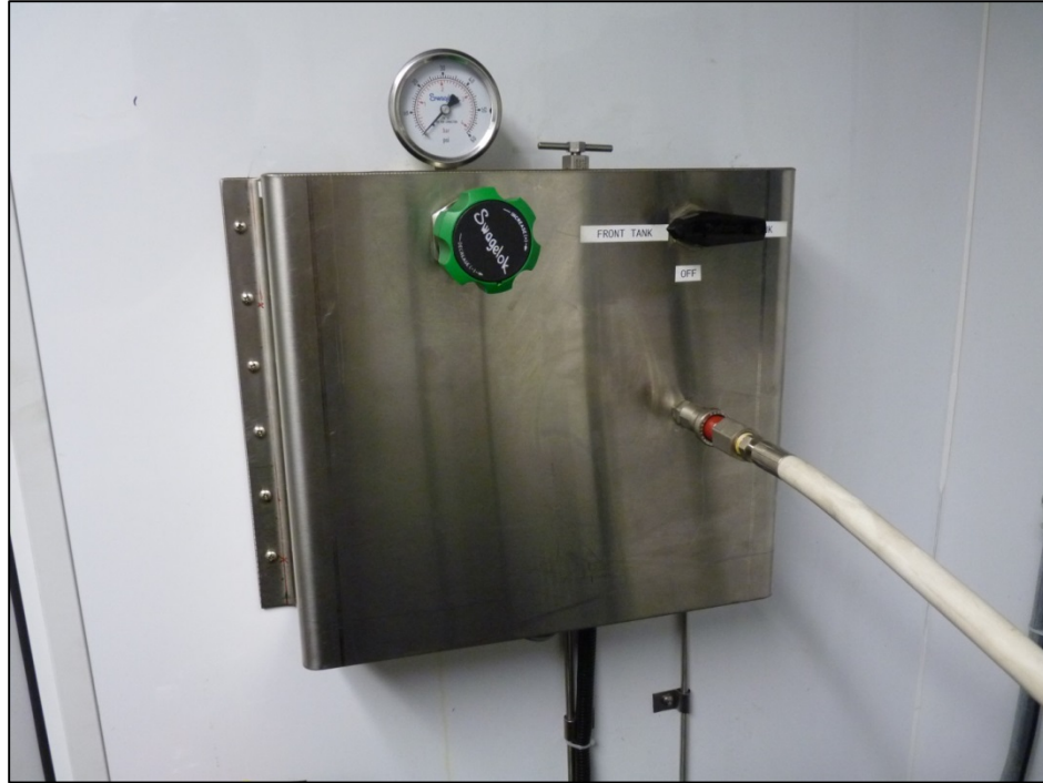
Figure 4.6: Fuel control panel in front test cell.
