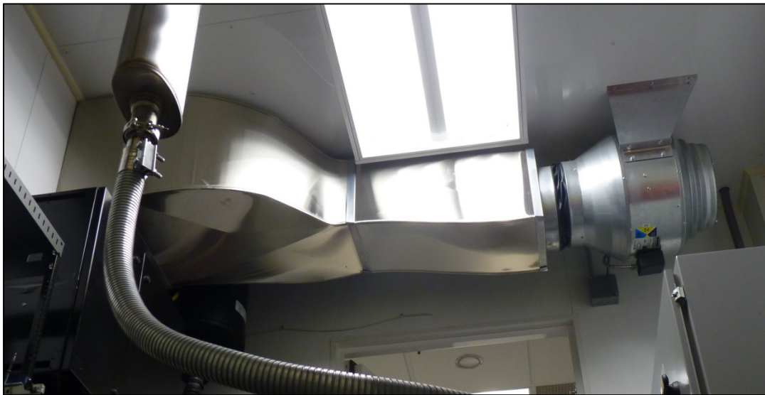
Figure 4.9: Picture of ventilation fan and ducting in rear test cell.
