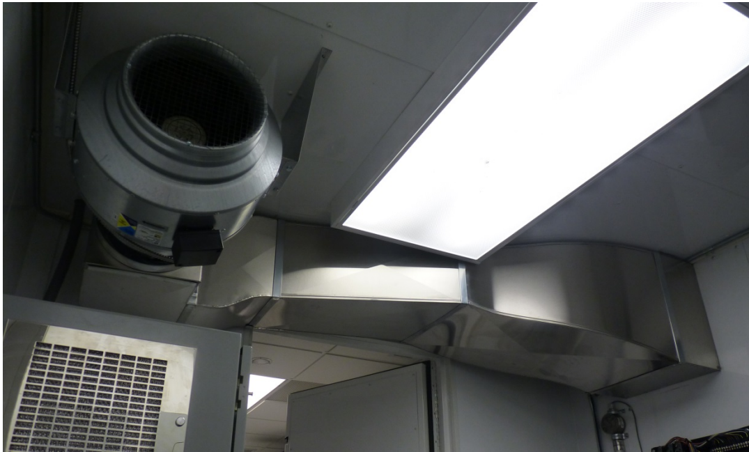
Figure 4.8: Picture of ventilation fan and ducting in front test cell.
