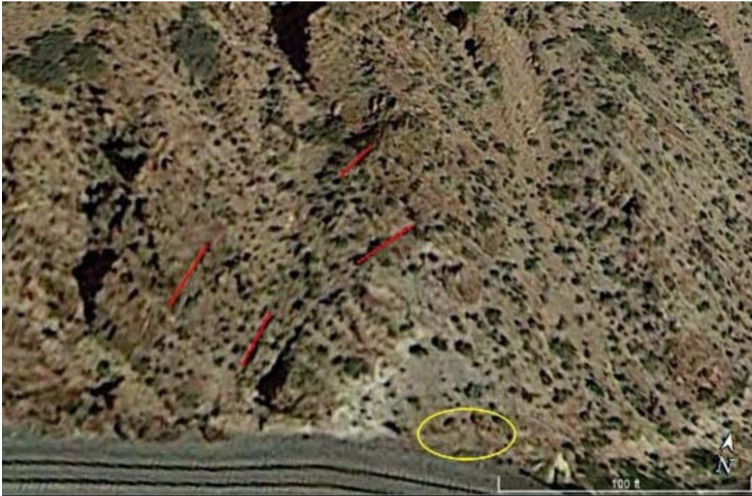
FIGURE 4-5: ZOOMED IN ORTHO-PHOTO OF SLIDE 3 FOR GEOLOGICAL CONDITION. THE RED LINES ARE FRACTURES IDENTIFIED IN THE SLOPE. THEY CAN BE MEASURED FOR LENGTH AND ASSESSED FOR WEATHERING. THE YELLOW OVAL IDENTIFIES FALLEN ROCK BLOCKS. THESE CAN BE MEASURED AND ASSESSED FOR THE "ROCKFALL EVENT" CATEGORY.
