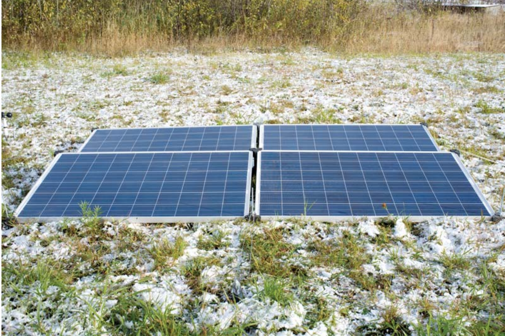
Figure 5.2: Assembled 1kW PV array with X-wire system. The 3-D printed components are shown in grey in Figure 2 are at the corners. The wiring forms an x-pattern beneath the modules.
