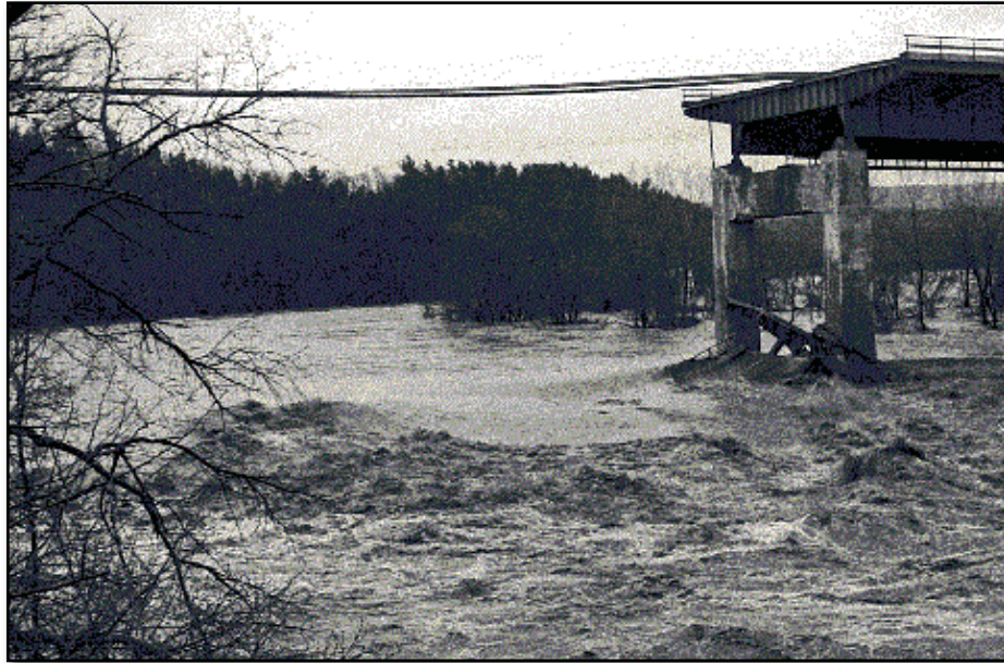
Figure 3. Schoharie Creek Bridge Collapse (Image Source http://water.usgs.gov/wid/images/NY.figure.id.3.gif , See Appendix-A for Permissions)
