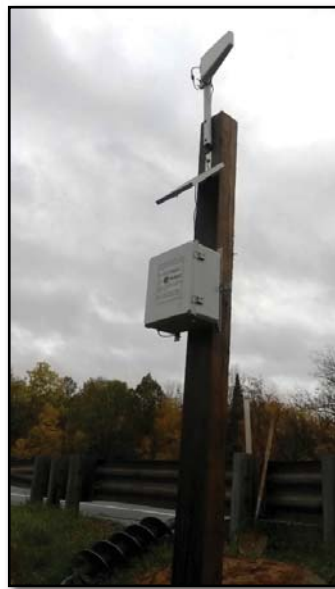
Figure 25. Assembled Based Station Installed in the Field (Image by Author)
