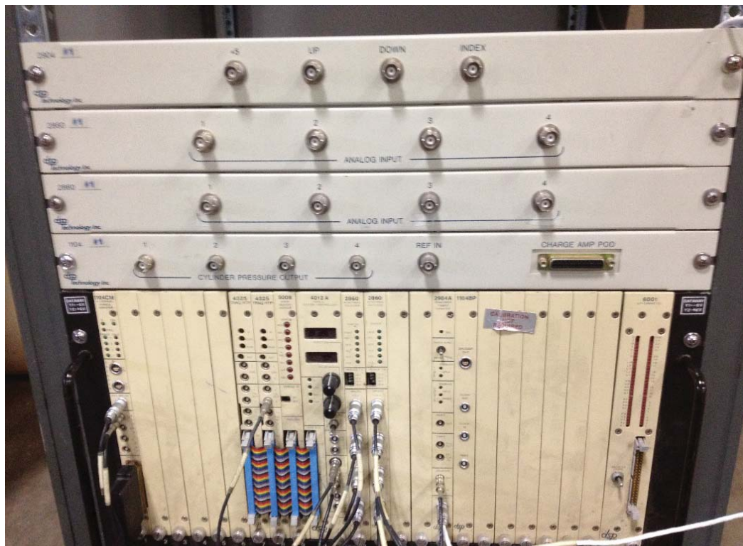
Figure 3-5: Test Cell ACAP System in 19 inch Cabinet
