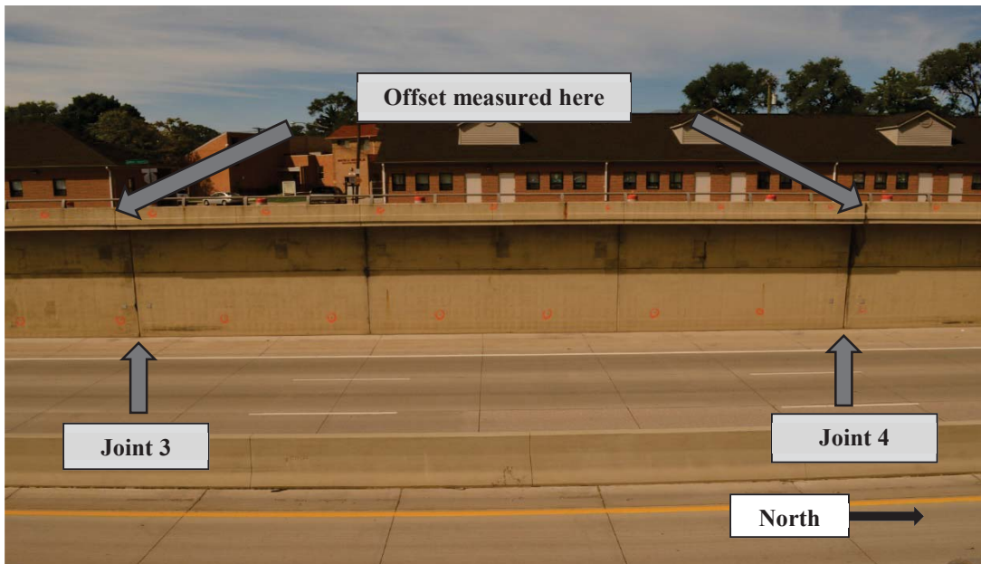
Figure 2-2 Retaining wall section at the Meyers site on M-10 Highway between Joint 3 and Joint 4. This is the section which experienced the most displacement relative to the adjacent walls.
