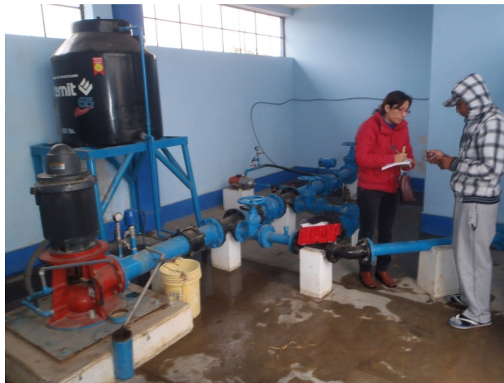
Figure 10 The Pump House Includes the Pump, Well Cap, and Chlorine Gas Injection System in Background (O'Neill, 2012)
