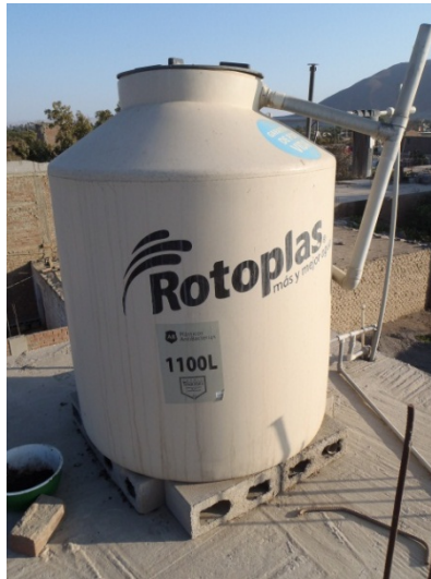
Figure 6 Residential Water Storage Tank on Rooftop (O'Neill, 2012)
