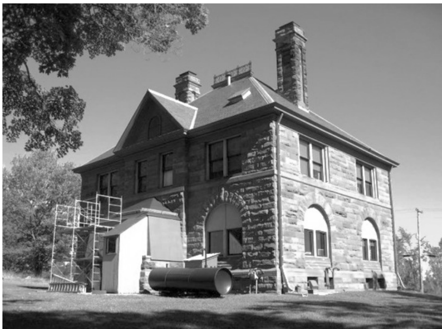
Figure 4.15: View of rear and south sides, Quincy Mining Company office. KNHP construction on the rear covered porch. Photograph by author, 2010.
