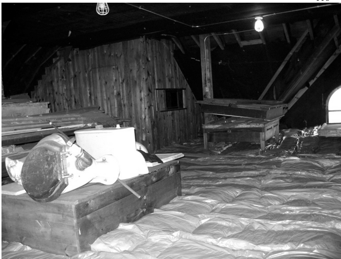
Figure 4.26: The attic space of the QMC office, with the floor covered in insulation. Note that there is a large drafting table in the rear of the photograph that could not be removed by the KNHP upon salvage of the office building in 2001. Photograph by author, 2010.
