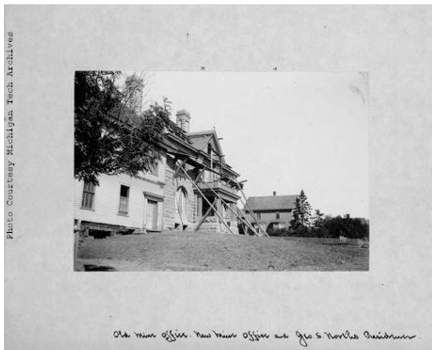
Figure 4.4: Detail of front façade of 1864 and 1897 QMC mine offices, looking north. Notice the stark contrast between the materials and construction of the old versus the new office. Image courtesy of MTUA/CCHC, image #:MS015.MI.2.217.
