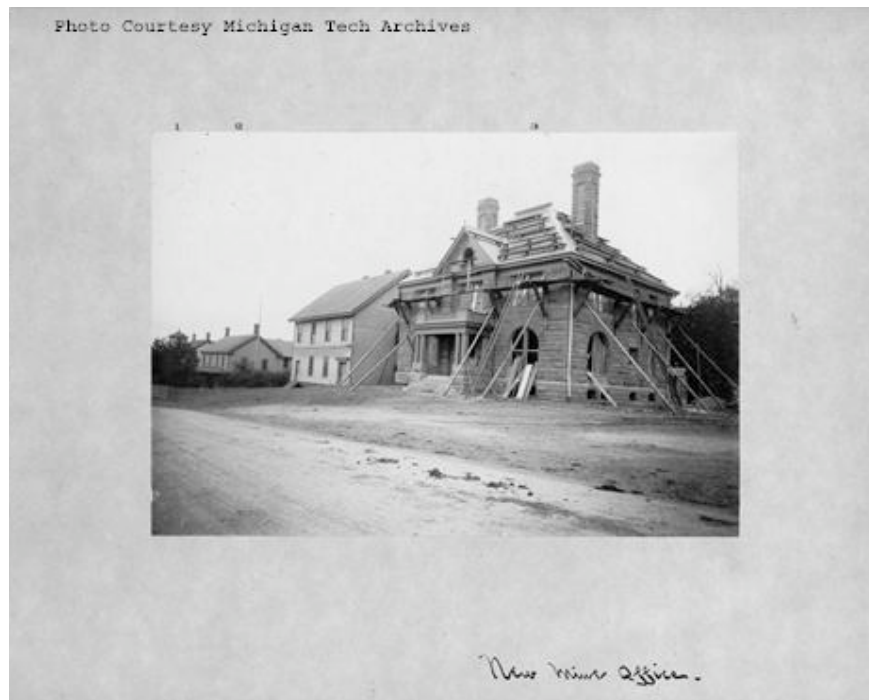
Figure 4.3: Construction of the 1897 QMC office with 1864 office in background, looking south from road. Image courtesy of MTUA/CCHC, image #:MS015.MI.2.218.
