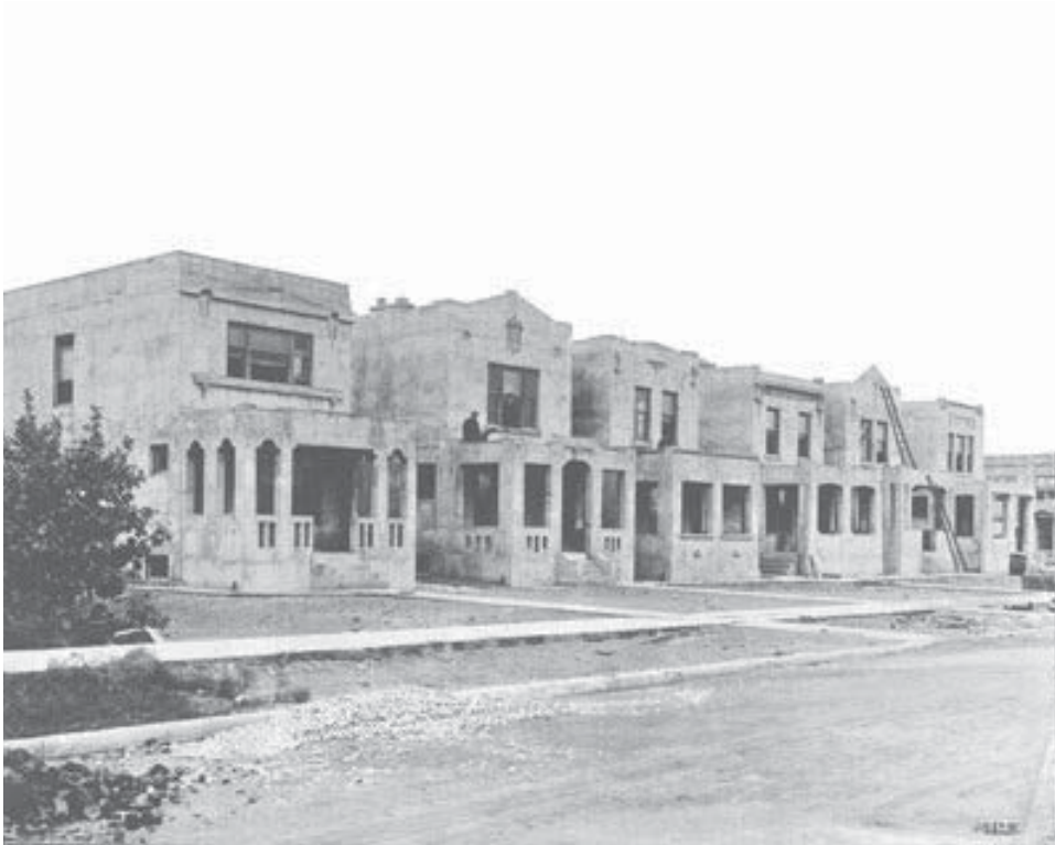
Figure 2.3 The Edison Concept concrete single-family homes under construction on Polk Street, 1912. Courtesy of Metal Forms Corporation.
