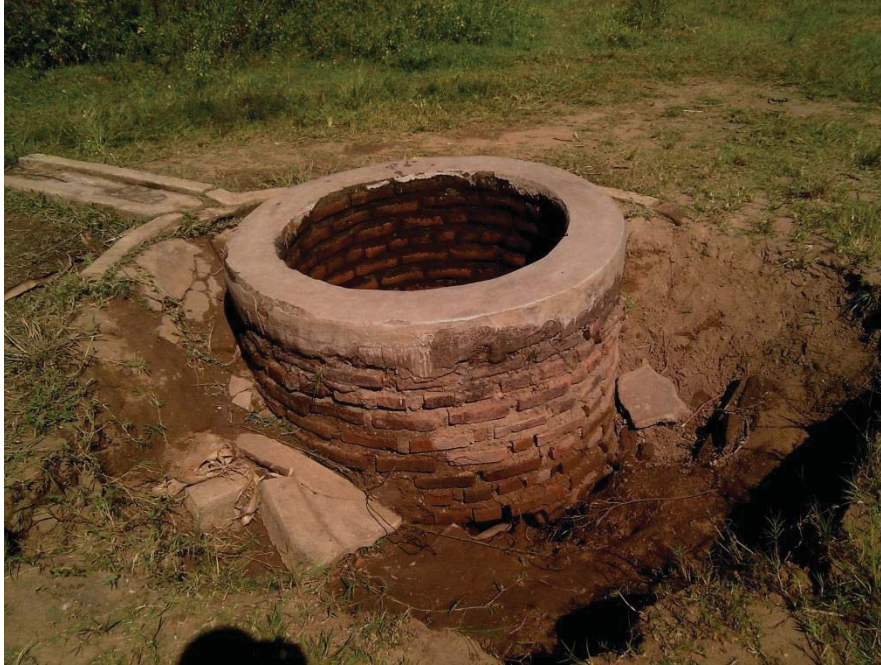
Figure 10: Deteriorating open well X
