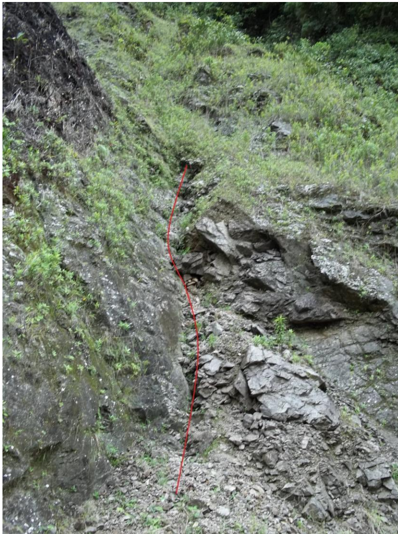
Fig.25: Outcrops along the road to Labonita village (Ros3). Intense fracturation of the material suggest the presence of a fault.
