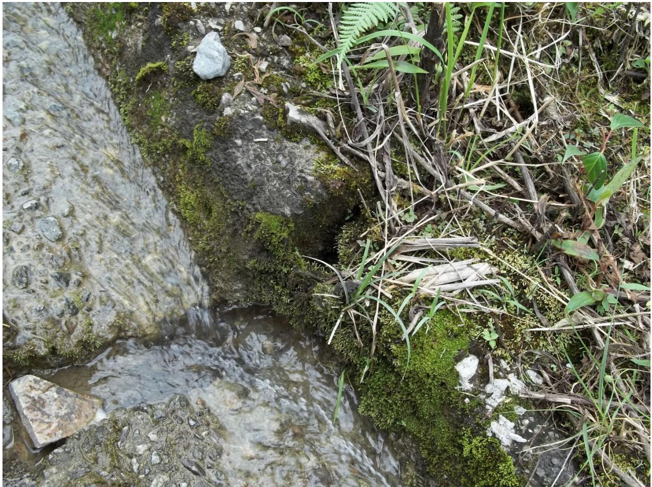
Fig.26: Deformation Ba8, particular of the concrete slab along the road limit (photo by M Balconi).
