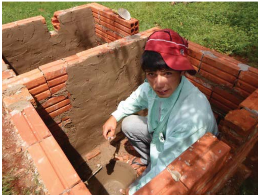
Figure 40: Ignacio putting layer of stucco on inside walls of vault. Photo by author.
