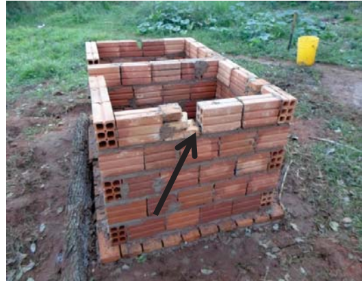
Figure 36: Opening on side of top layer of bricks for urine diversion tubing. Photo by author.
