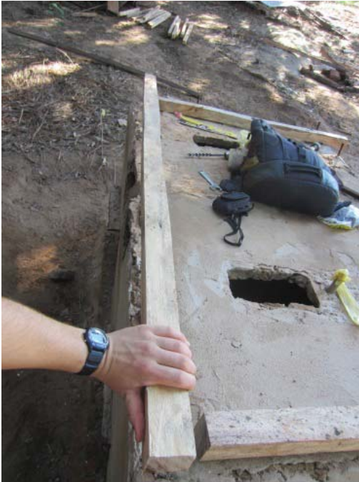
Figure 51: Lining up footer with outside edge of vault to ensure a straight wall after drilling. Photo by author.
