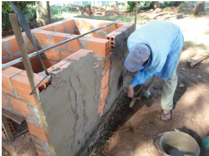
Figure 46: Author's neighbor is 'throwing' stucco on to outside walls of vaults. Photo by author.
