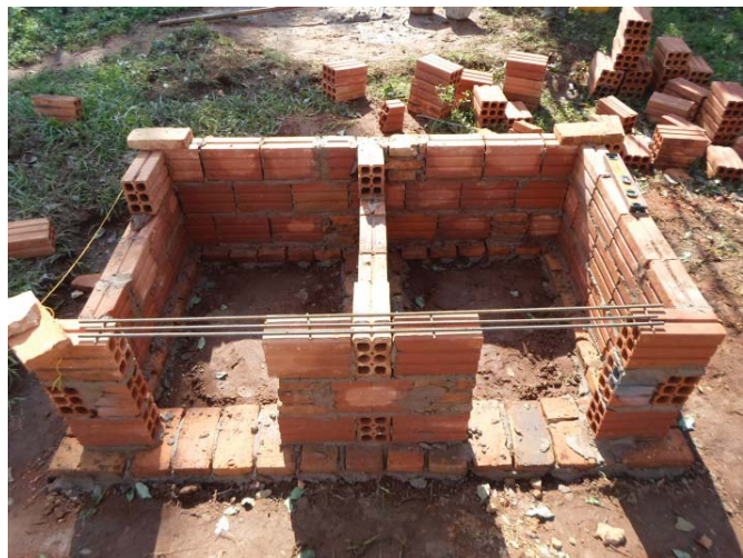
Figure 31: Completed first three levels of bricks. Three lengths of rebar are laid over the door openings to add support to the structure. Photo by author.
