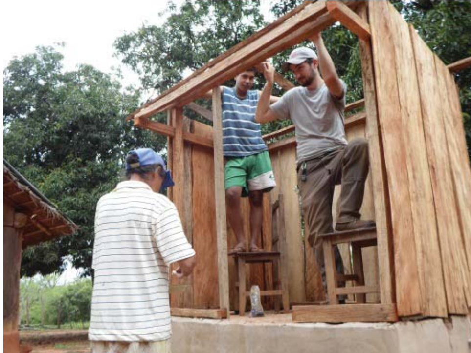
Figure 63: Attaching planks to complete walls of latrine housing structure. Photo by author.
