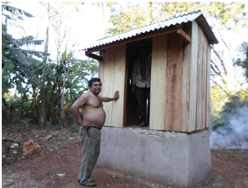
Figure 13: Completion of first commission latrine. The stairs were added later by the owner. Photo by author.
