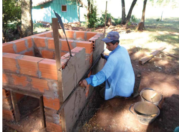
Figure 47: Author's neighbor Io smoothing stucco with long metal ruler. Photo by author.
