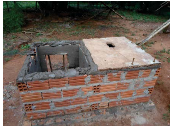
Figure 43: Preparing top of vault with mortar for placement of left loza. The right loza has already been placed. Photo by author.
