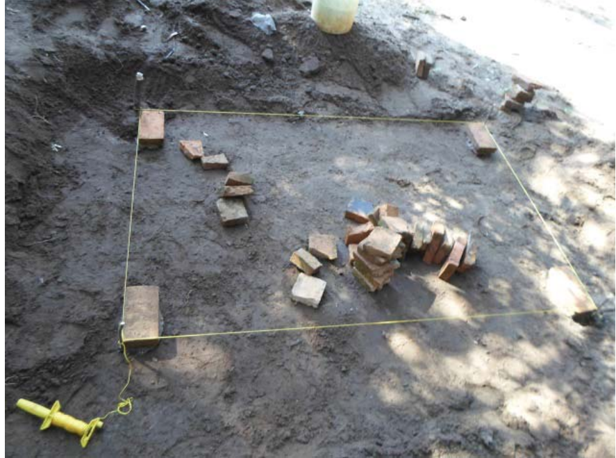
Figure 24: String strung between stakes to show placement of base level of bricks. Photo by author.
