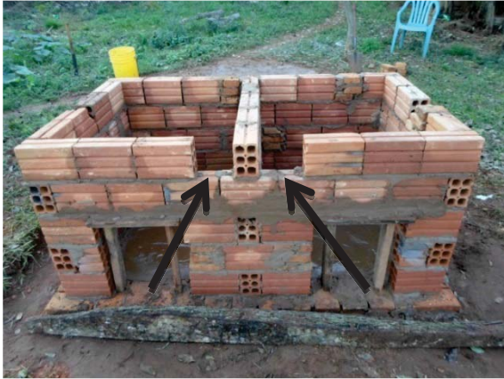
Figure 37: Openings in back for ventilation tubes on the final layer of bricks. Photo by author.
