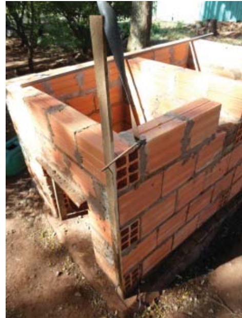
Figure 45: Stucco thickness guide attached to outside corner of vault. Photo by author.
