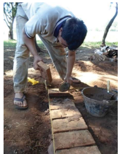
Figure 25: Base level of bricks being laid using string lines. Photo by author.
