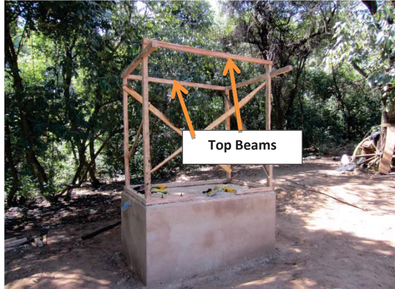
Figure 58: Front and back top beams placed on latrine structure. Photo by author.
