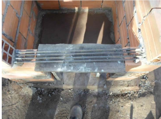
Figure 32: Rebar placed over door opening before bricks were laid. Photo by author.
