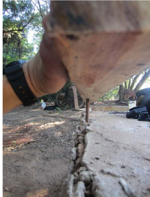
Figure 52: Lining up threaded bars in center of footer to mark for drilling. Photo by author.
