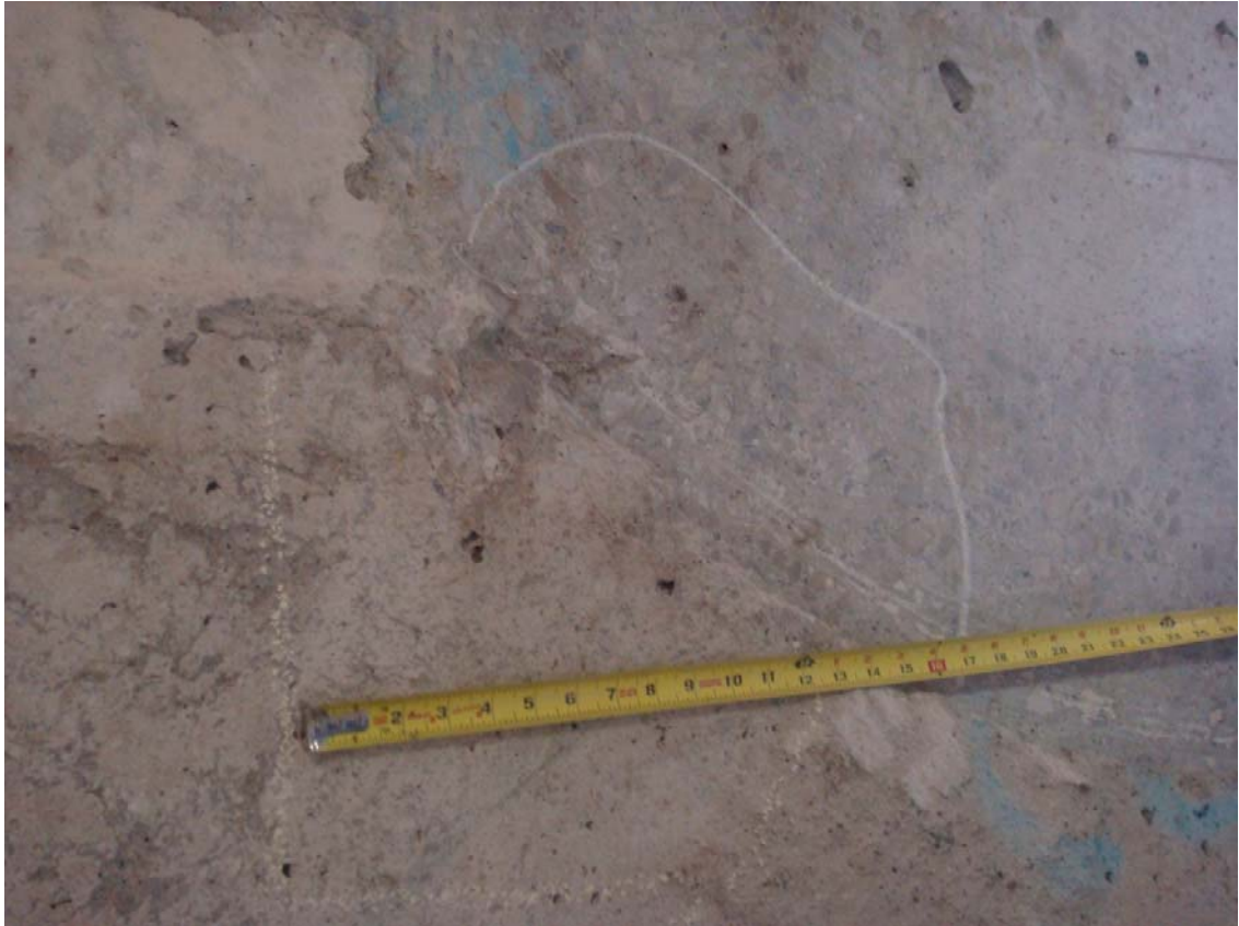
Figure 6.23 Visible condition of the concrete surface at location E1.
