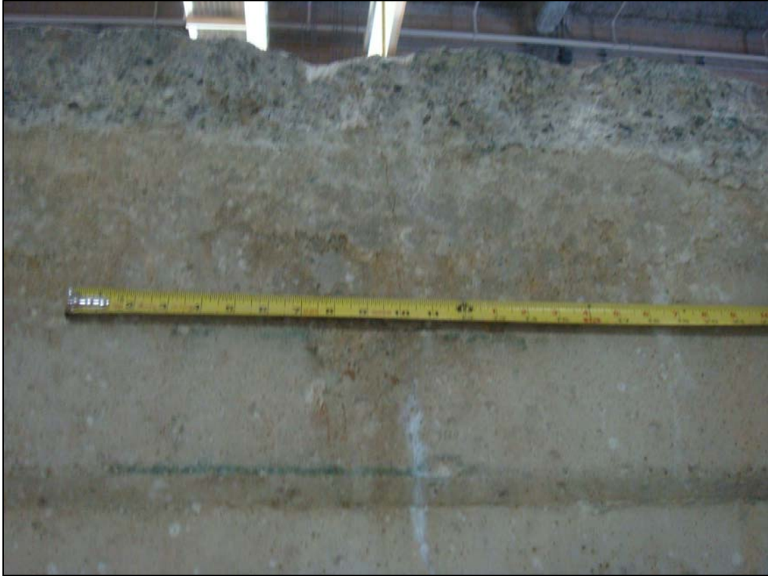
Figure 6.31 Visible surface crusting on the concrete surface at location E3.
