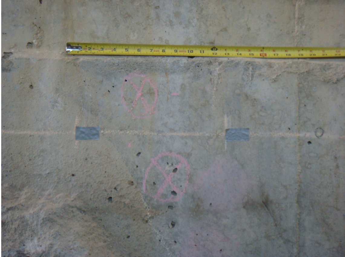
Figure 6.14 Visible condition of the concrete surface at the location W2.
