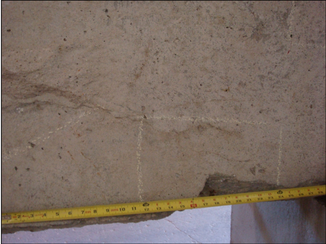
Figure 6.27 Visible condition of the concrete surface at the location E2.
