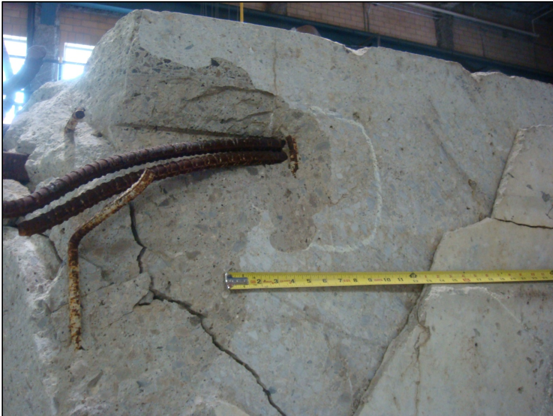
Figure 6.35 Visible condition of the concrete surface and mild steel at the location E4.
