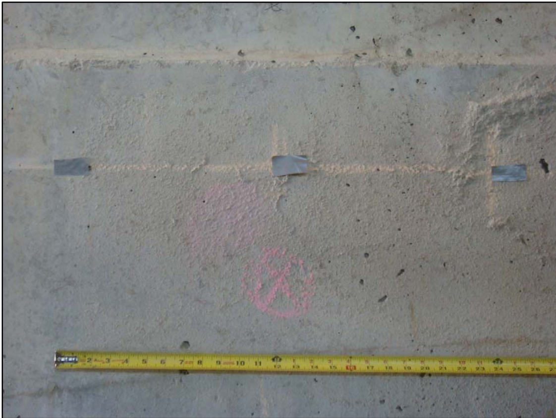
Figure 6.41 Location W4 with no delaminations.
