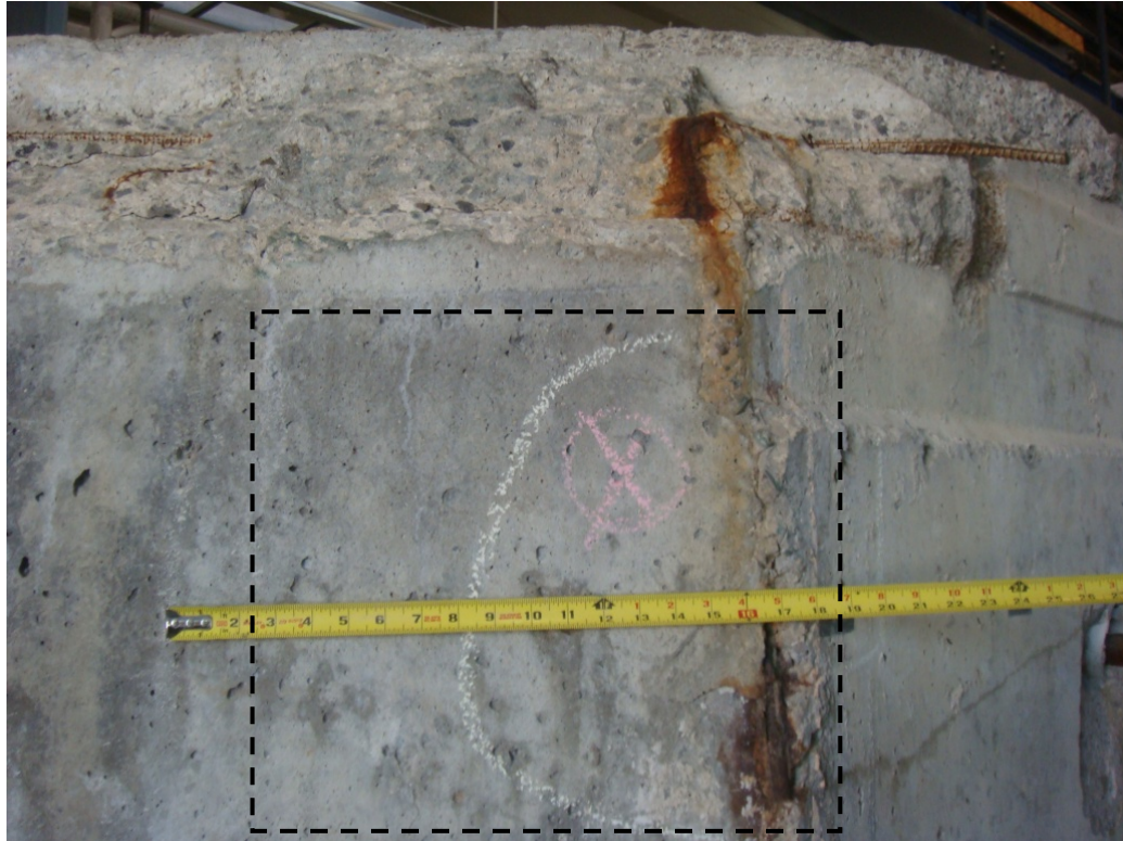
Figure 6.10 Visible condition of the concrete surface at the location W1.
