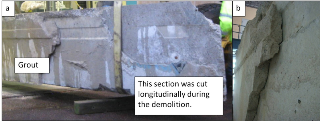
Figure 6.22 (a) Side of the Silverbell Bridge beam showing the grouted segment and the section that was cut during the demolition (b) grout that is delaminated from the precast section.
