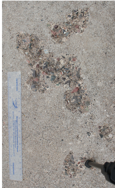
Figure 4.14: Picture of Scaling in Test 4
