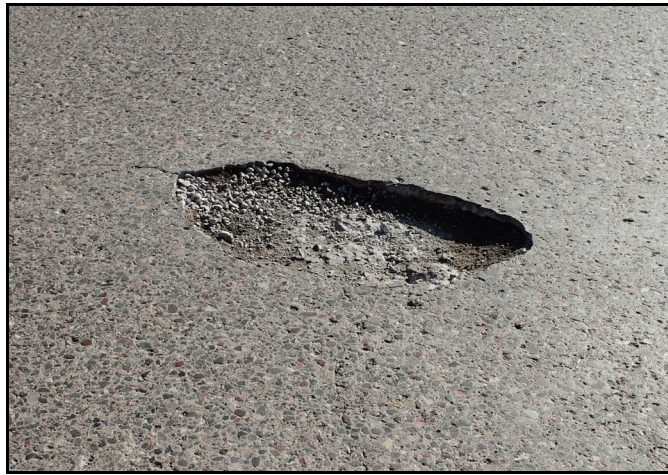
Figure 2.2: An Example of a Spall
