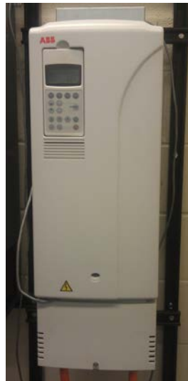
Figure 3.2: ABB Variable Frequency Drive
