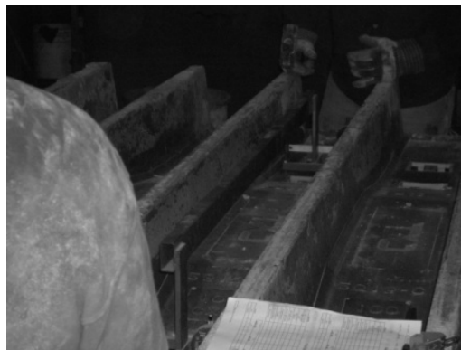
Figure 37: Workers checking rail cant and gauge of tie form using jig equipped with dial gauges
