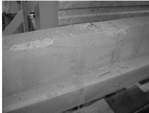
Figure 79: Cracking in bottom flange of beam outlined in black marker occurs prior to complete failure of beam
