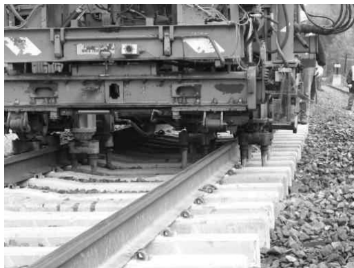
Figure 21: First round of tamping, consolidation restricted to rail seat region (Peters and Mattson 2003)
