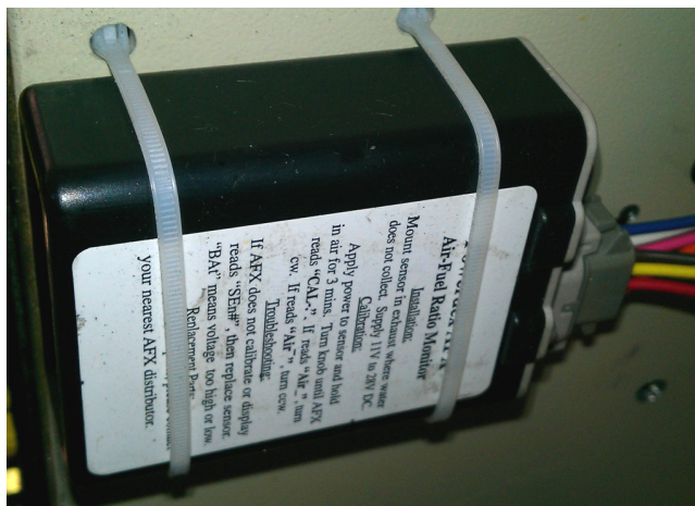
Figure 3.10: Powerdex AFX controller used to monitor relative air/fuel ratio.
