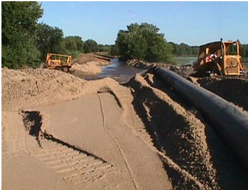
Figure 2.1: Levee Repair, Green Island Levee District (Figure Courtesy of U. S. Army Corps of Engineers, Rock Island District [Date Unknown] Unpublished Photograph) (Documentation can be found in Appendix E)
