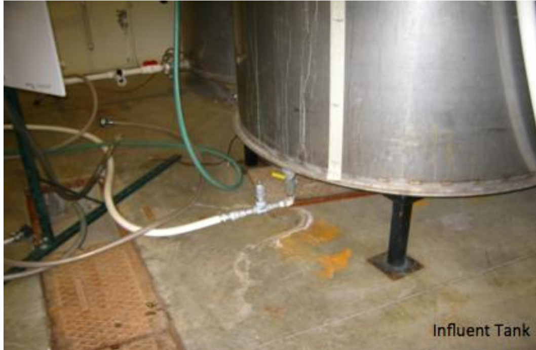
Figure 5. Stainless Steel Tank for Influent Storage
