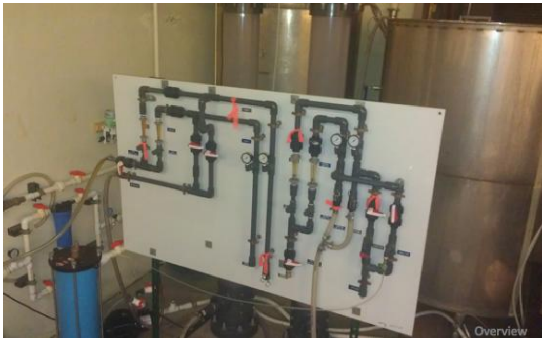
Figure 4. Overview of Direct Filtration Unit
