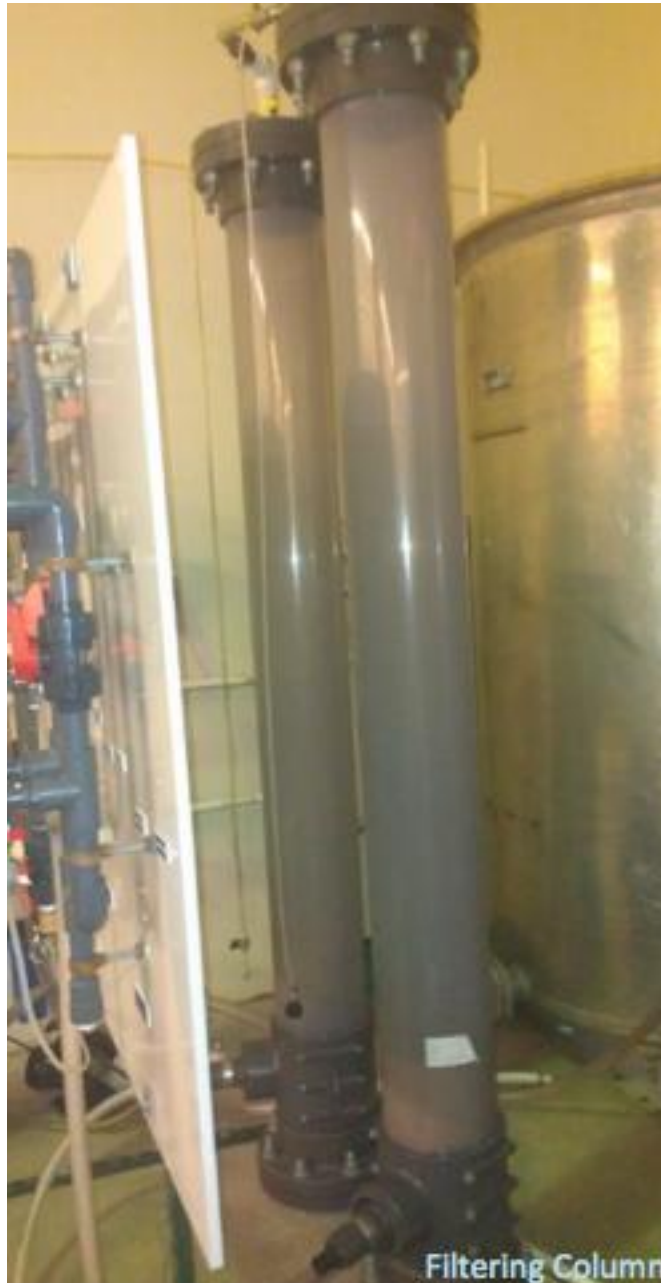
Figure 10. Sand Filtration Unit
