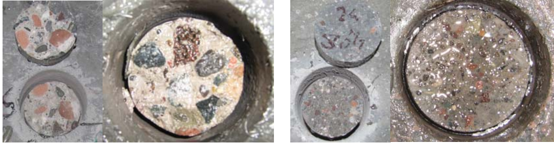
a) C: Concrete failure
