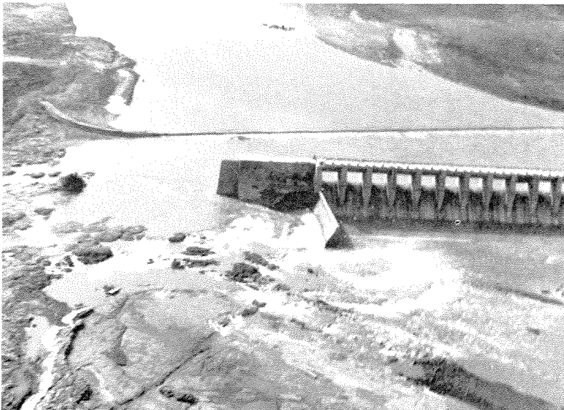
Fig. 3 Aerial photograph of the collapsed Machhu-2 dam. The earthen flank to the right of the masonry dam was washed away on 11 August 1979 and even 3 days after the disaster the water continues to rush through the breached portion. (Photo by courtesy of the Information Department of the Government of Gujarat at Rajkot.)
