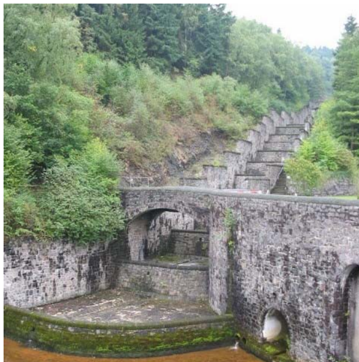
Sorpe dam pooled stepped spillway in September 2003 (Courtesy of Dr Carlos GONZALEZ)
