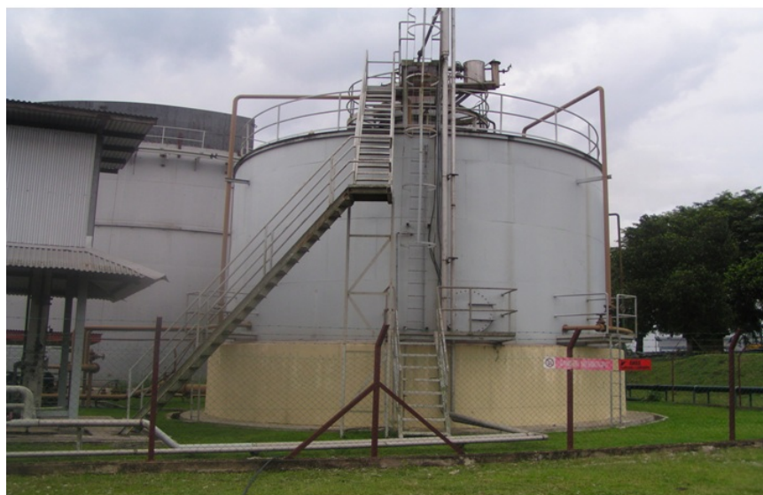
Fig. 2: The 500 m 3 semi-commercial scale closed anaerobic digester dedicated for methane recovery for renewable energy research belongs to UPM-KIT-FELDA joint R&D collaboration in Serting Hilir Palm Oil Mill, Negeri Sembilan, Malaysia.
