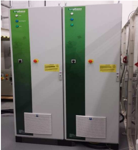
Fig. 10. Controllable Power and Voltage Source (Triphase).
