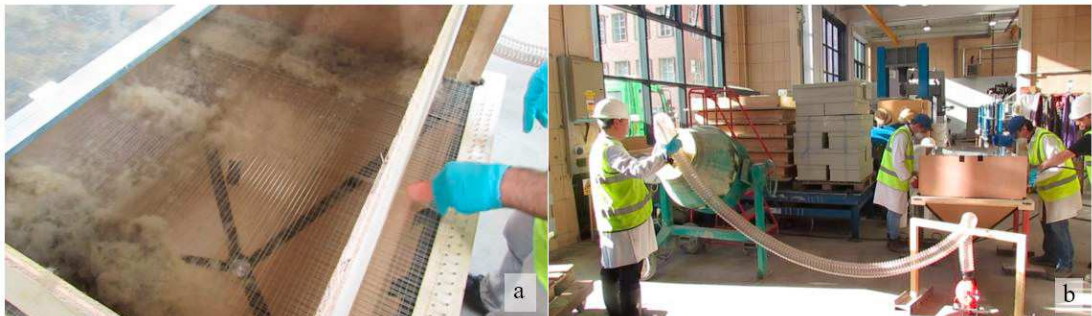
Fig. 4. Fibres integration stages (a) strings being manually excited; (b) fibres being integrated into the concrete mix.
