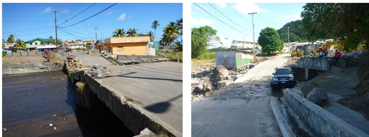
Figure 7: Photographs showing flooding and bridge damage in St. Vincent used in the workshop scenario (photo credits: Anna Hicks, BGS © NERC).
